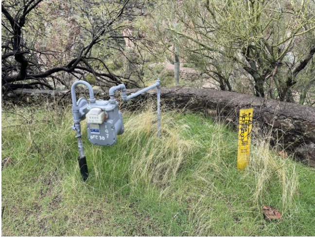
Photo 13: Natural gas pipeline and marker.
