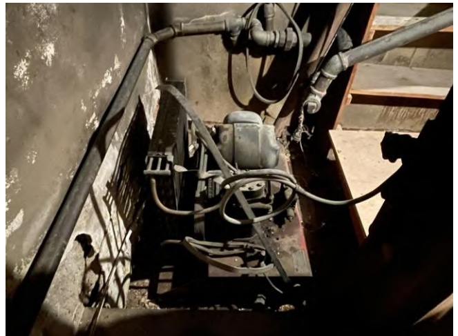
Photo 24: Compressor in the kitchen storage room of Building 1.
