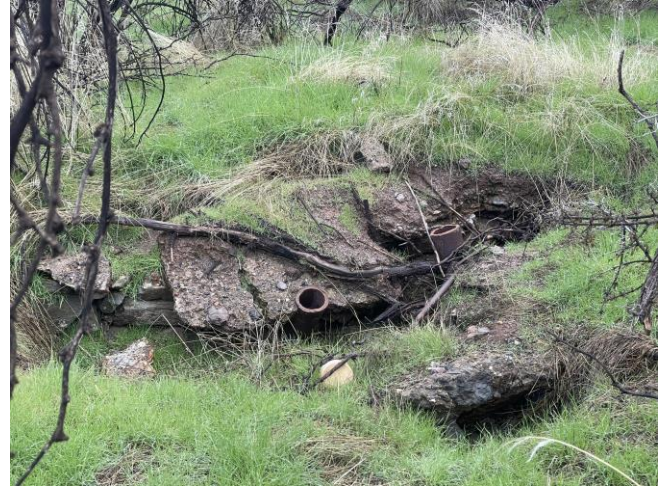
Photo 14: Possible former septic, near Building 9.
