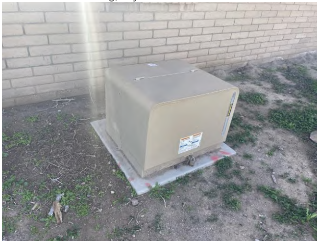
Photo 9: Pad-mounted transformer, located outside the Town Hall building.
