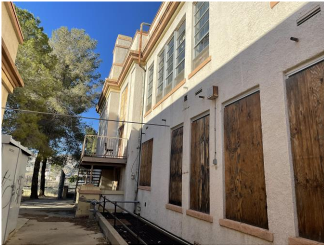
Photo 7: Southeast, rear face of Inspiration school, showing boarded windows.
