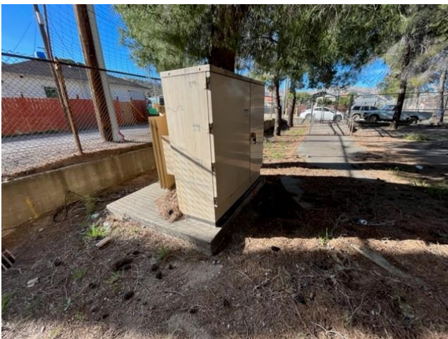
Photo 23: Transformer located next to right side
